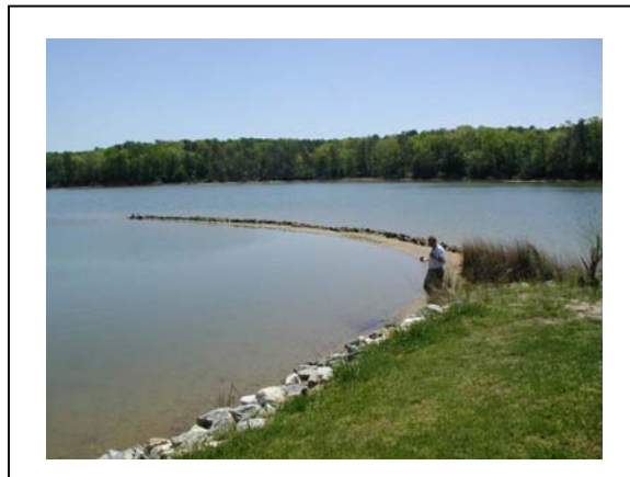
Figure 8. If upland revetments sever the landward end of a marsh spit, then marsh toe protection structures may not reverse the trend of “drowning” spit marshes. This is the only case where the revetment was not at all effective for erosion control (LA06).
