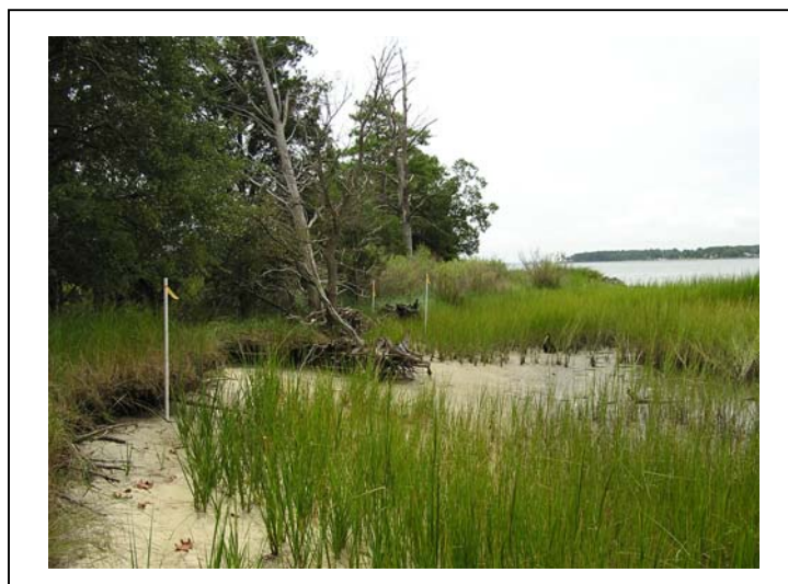
Figure 6. Spots of upland bank erosion were observed where the crest height of the marsh toe protection structure was less than +1 ft MHW in a medium energy setting. The white stakes indicate a proposed upland revetment (MA05). Raising the crest height of the marsh toe protection structure was encouraged instead to preserve the natural connections between the upland and wetland habitats.
